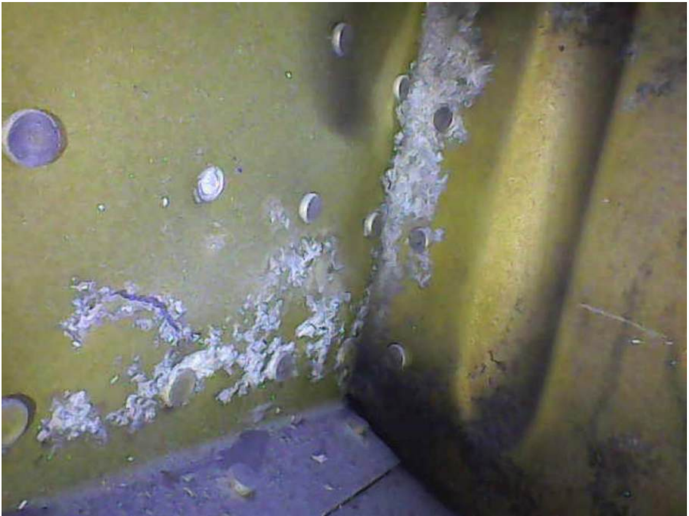
CORROSION ON AFT SIDE OF FORWARD WING SPAR AND INBOARD WING RIB
